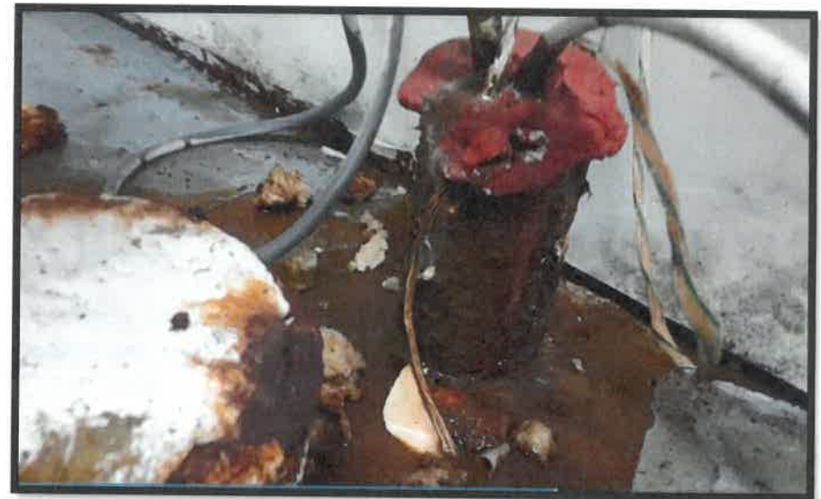
Water spews out of data port conduit during rainstorm April 2022
