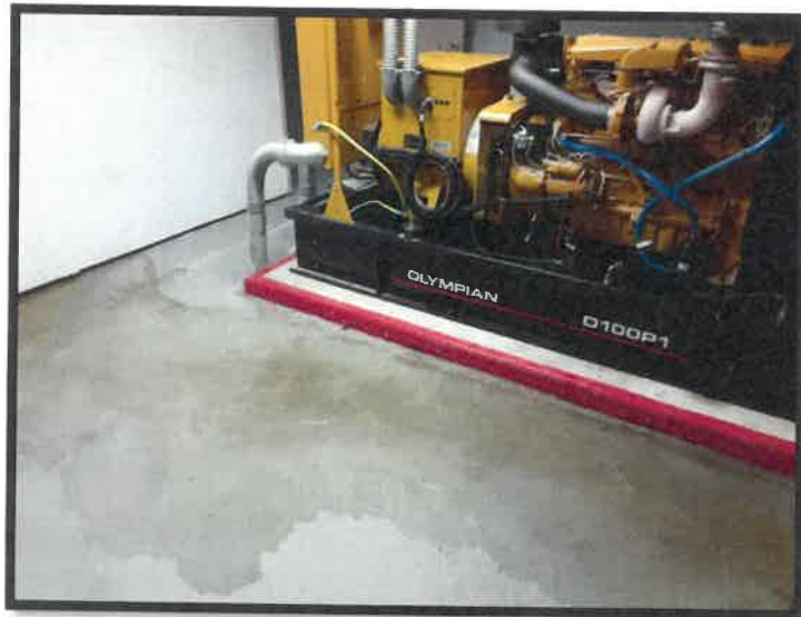
Flooded LEDU Basement shop vacuumed during each rainstorm. Water flows directly towards an emergency generator.
